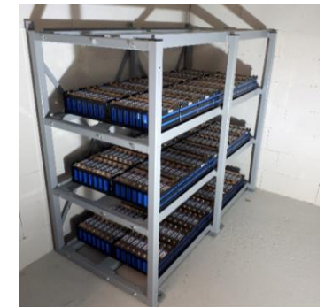
37.5 KWh battery bank
